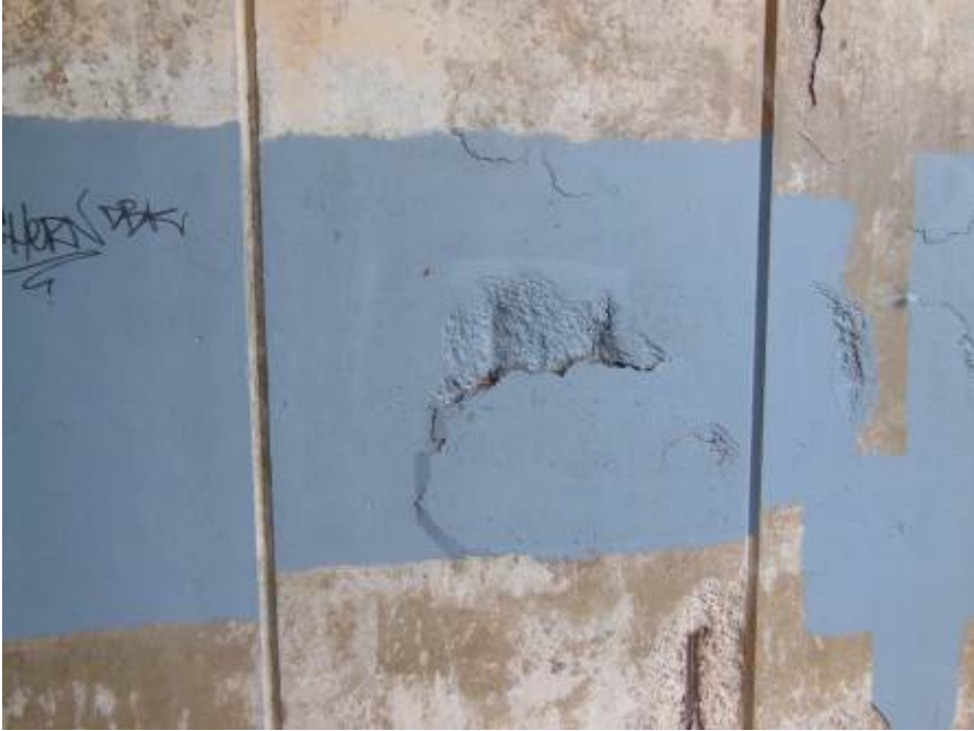
Figure 44 - Spalling to the abutments
