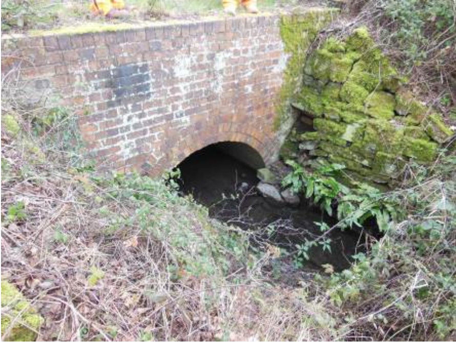
Figure 30 – Culvert B: view North side of line: collapsing wingwalls
