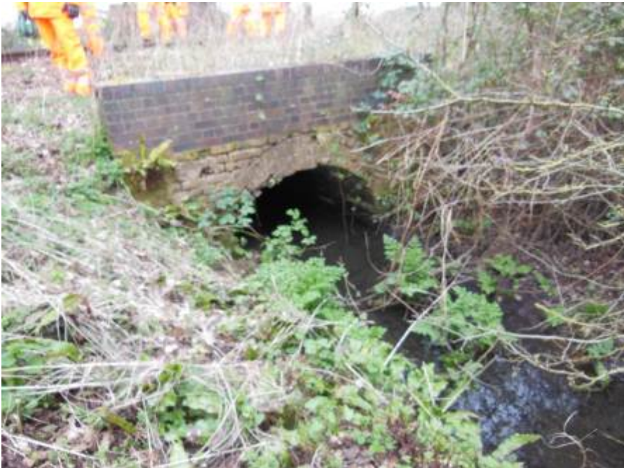
Figure 29 – Culvert B: view South side of line: spalled masonry and open joints visible
