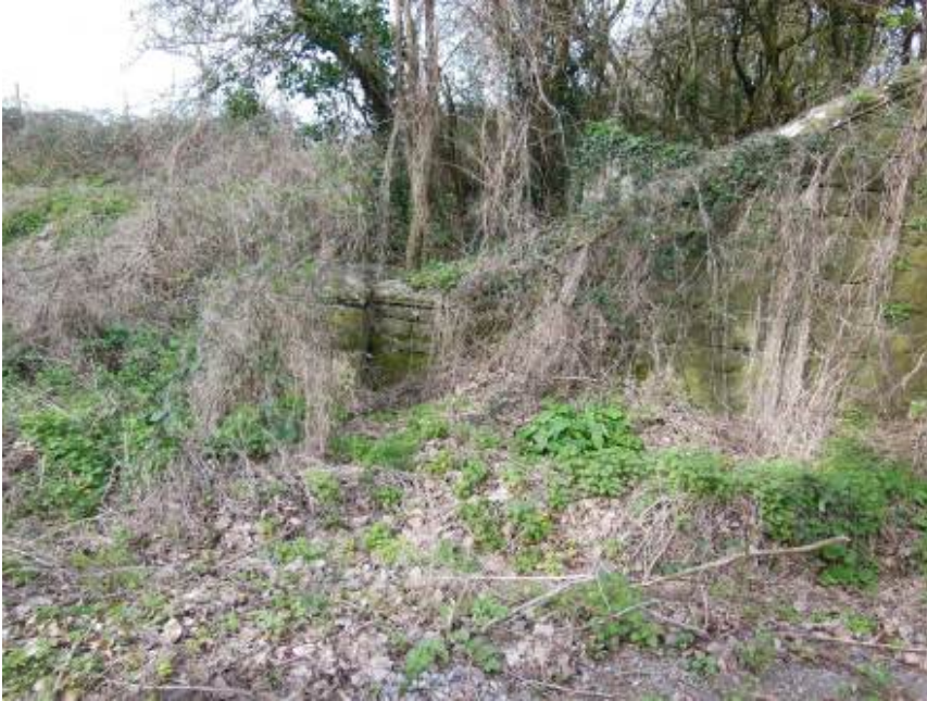
Figure 36 - Wing wall fractured joints on coping stones – Marsh Lane
