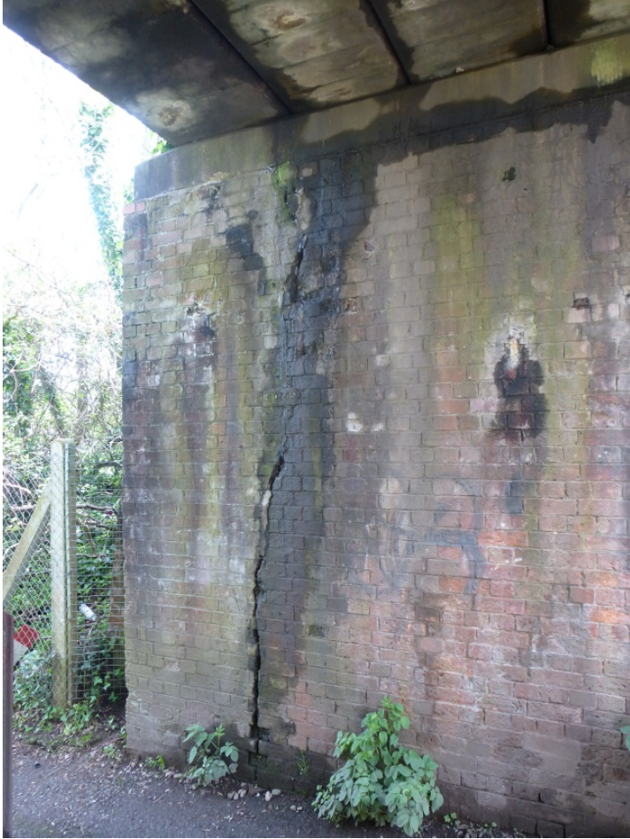
Figure 51 – Spalling and full height vertical fracture in low mileage abutment (<25mm). Stepped hairline fracture visible at top of the abutment.
