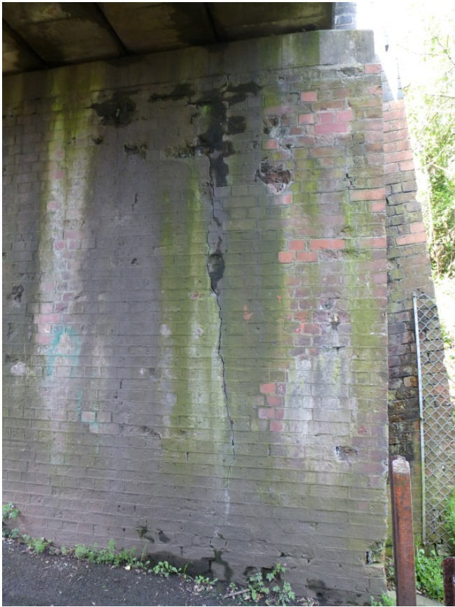
Figure 50 – Spalling and hairline full height fracture (<5mm) to high mileage abutment. Vegetation requires removal from structure and treating to prevent regrowth.
