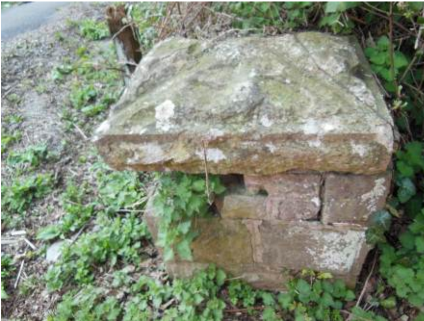
Figure 37 - Stones under newel cap missing
