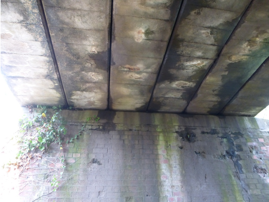
Figure 48 – Bridge soffit: isolated spalling and visible corrosion
