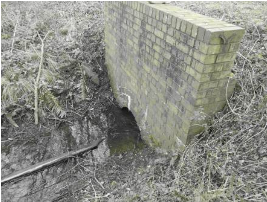
Figure 32 - Culvert C: channel silted up
