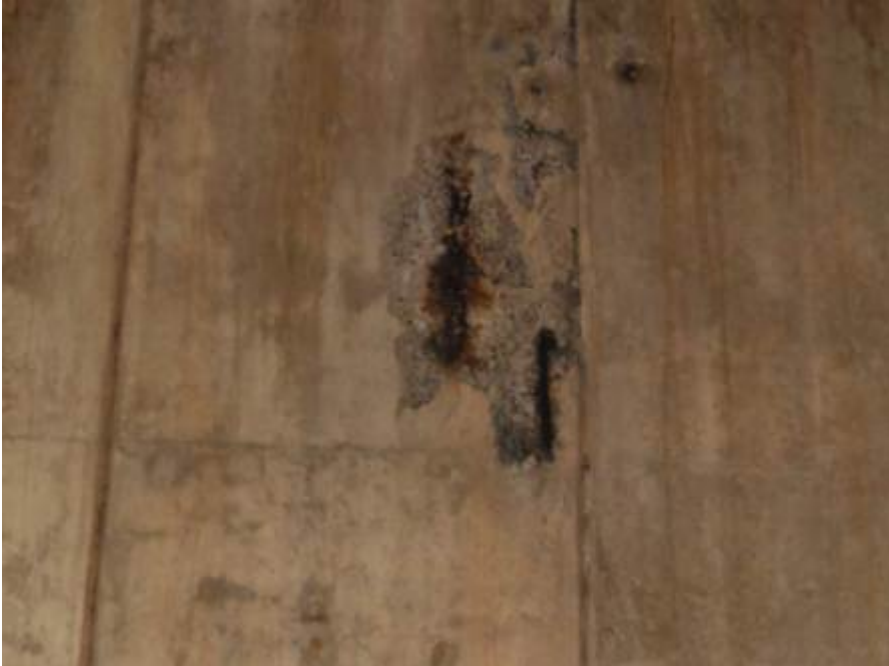
Figure 42 – Isolated areas of spalling and visible corroded reinforcing bar
