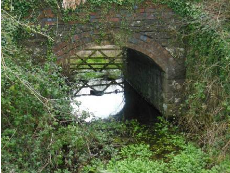
Figure 40 - Cattle creep: open joints visible in the arch rings and spandrel wall
