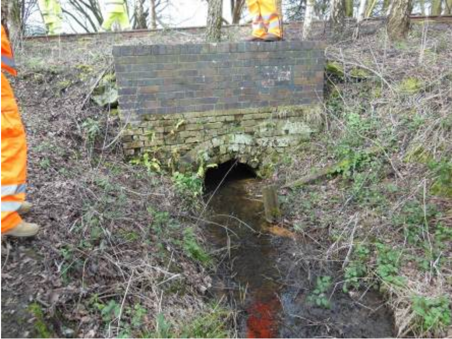
Figure 31 - Culvert C: spalled masonry and silted up channel
