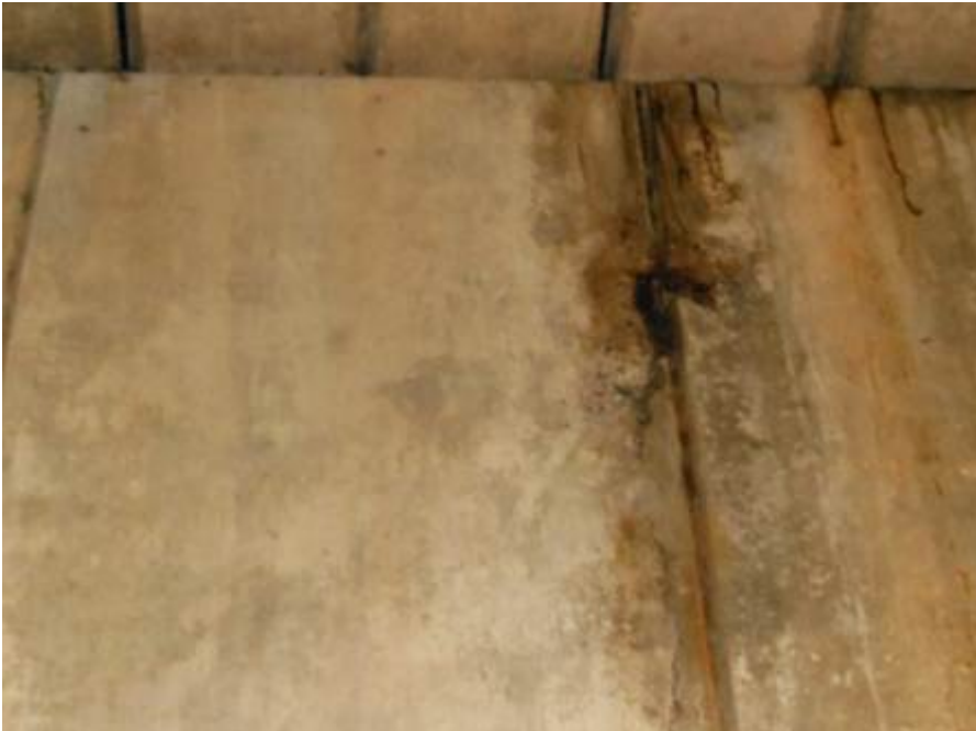
Figure 43 – Isolated areas of spalling and visible corroded reinforcing bar
