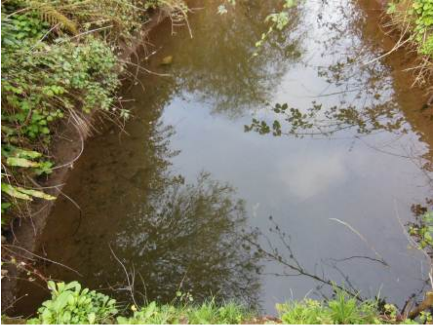
Figure 38 - Culvert adjacent to overbridge requires inspection
