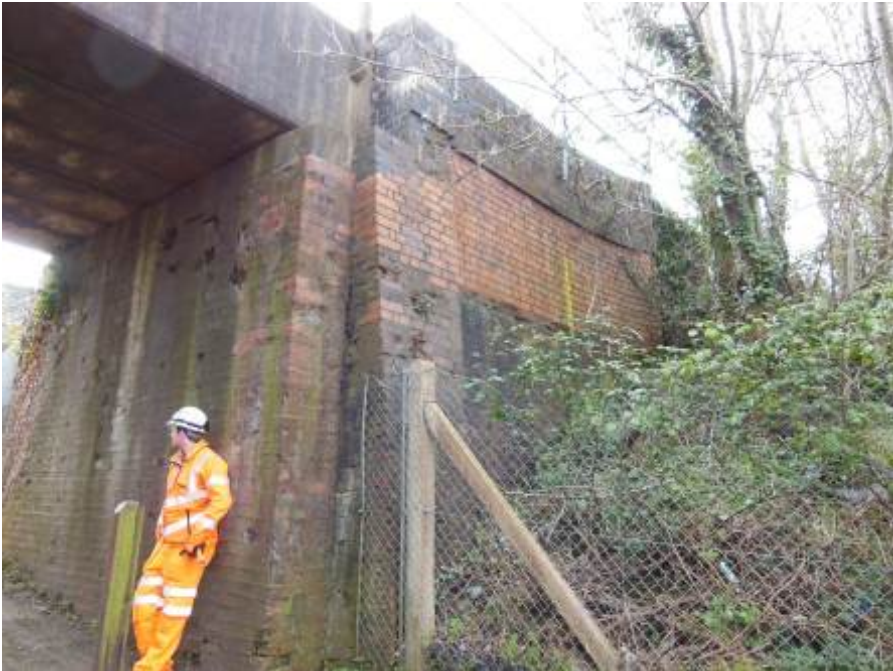
Figure 49 – Spalling to masonry on buttress and abutments
